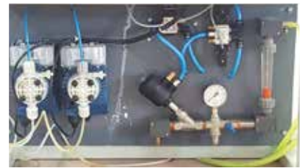
Compound Dosing System
